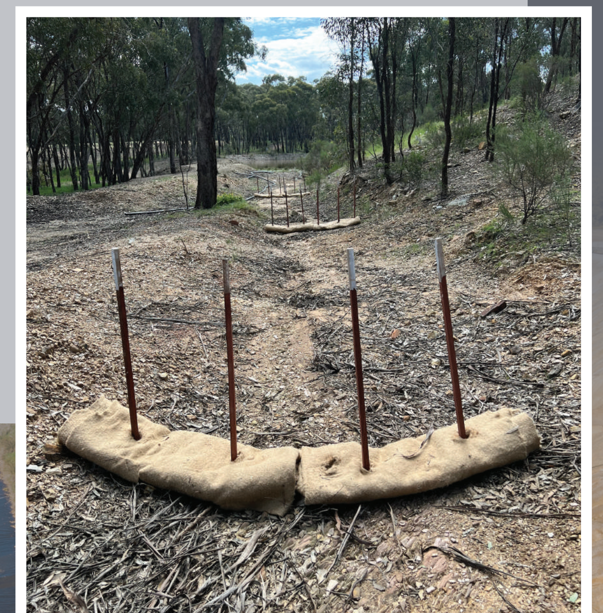
Right: Coir logs installed in drainage channels. Below: The ASTER plant treats residual cyanide species in process water.
